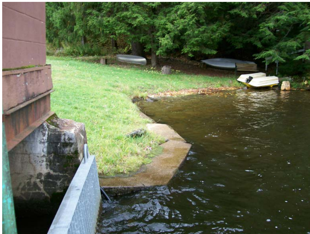
Photo 17 - Upstream slope at right abutment. Note repairs made to previously reported erosion.
