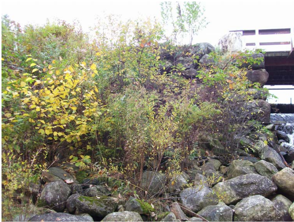
Photo 11 - Vegetation growing within rip rap surface on the downstream slope adjacent to the spillway.
