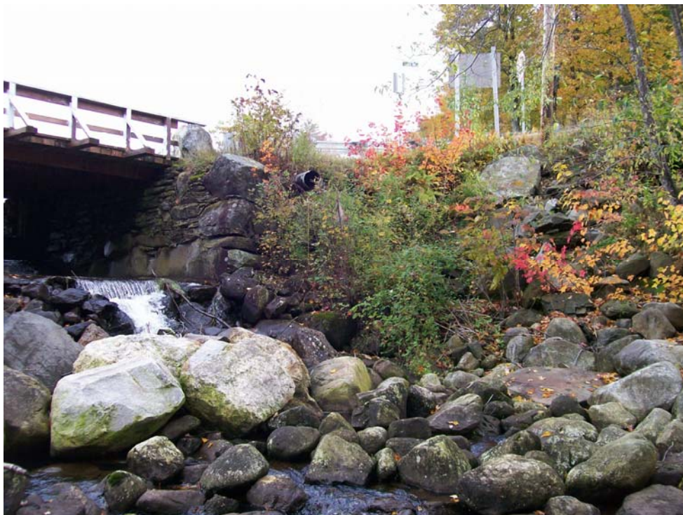
Photo 12 - Vegetation growing within rip rap surface on the downstream slope at the left abutment.
