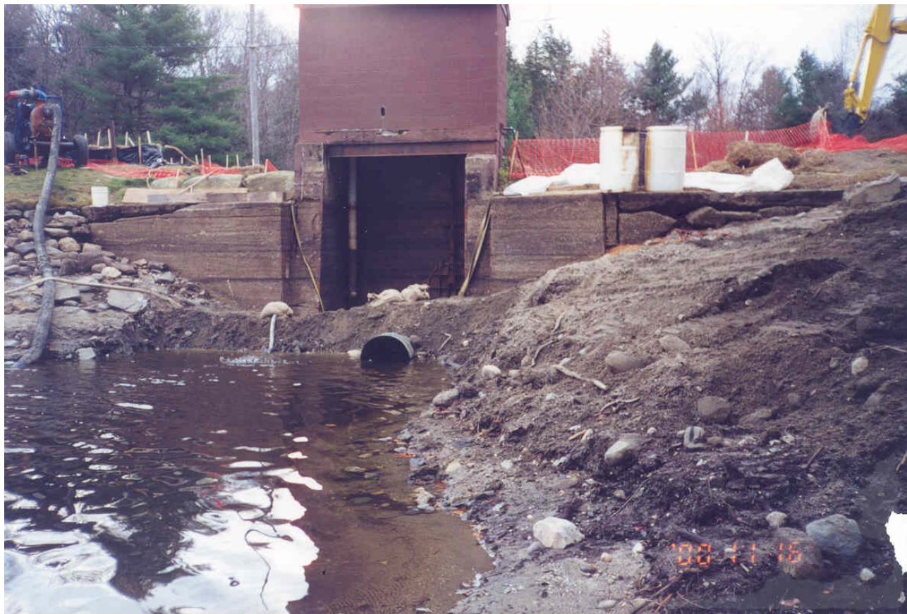
Photo 23 - Photo taken during the construction of the improvents at Hammond Pond Dam in 2000. This photo shows that the cracks in the concrete to the left and right of the gatehouse are at locations that are not part of the gatehouse foundation and do not present a threat to the structural integrity of the gatehouse, or the embankment.
